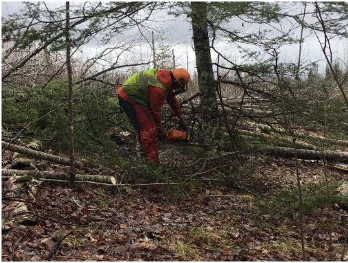
The clearing process involves both hand-cutting and machine-cutting trees at their base.
