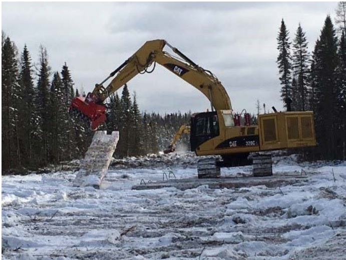
Excavator clearing trees, working off of timber mats to lessen impact in sensitive/wet areas.
